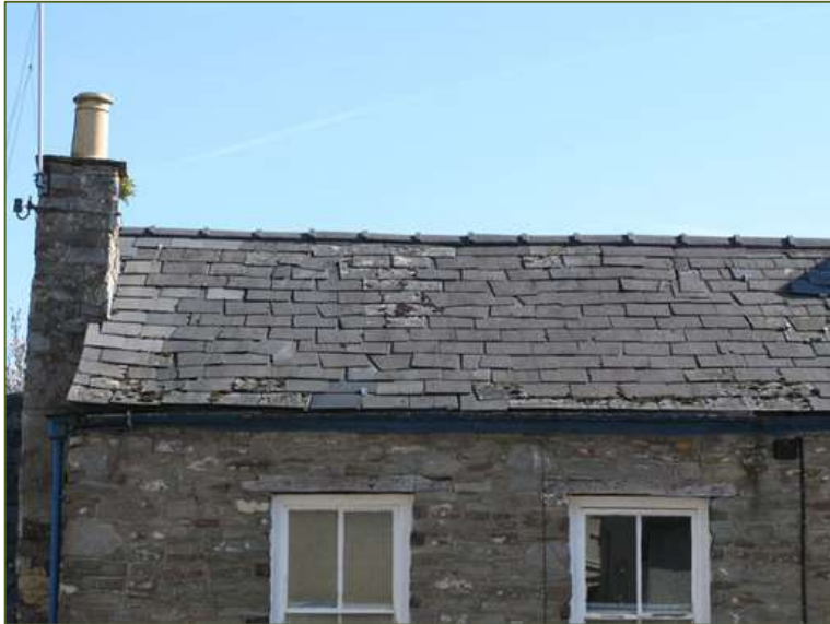
Examples of loose slates, leaking down-pipes and blocked gutters
