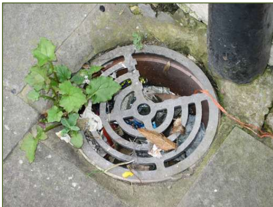
Blocked drains and effect of elevated ground level
